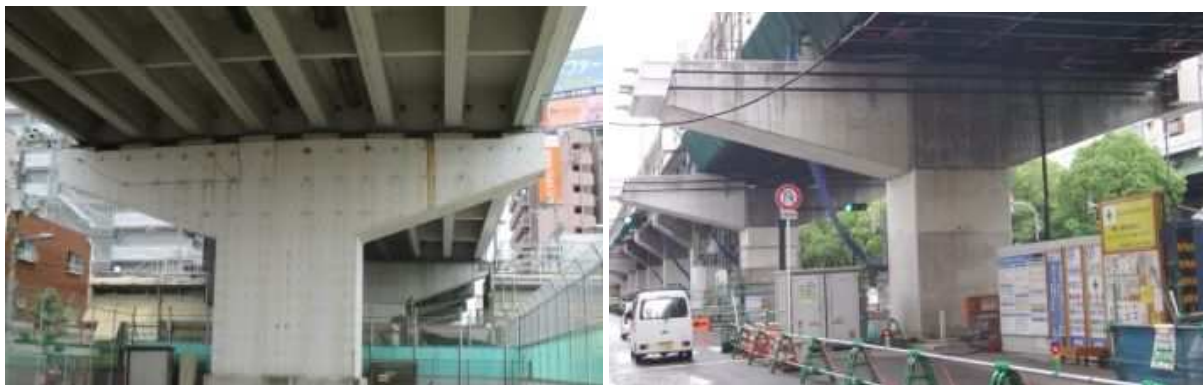
(a) Steel plate bonding (b) External cable system Figure 1. Examples of strengthening of PC beams of ASR-affected piers.
